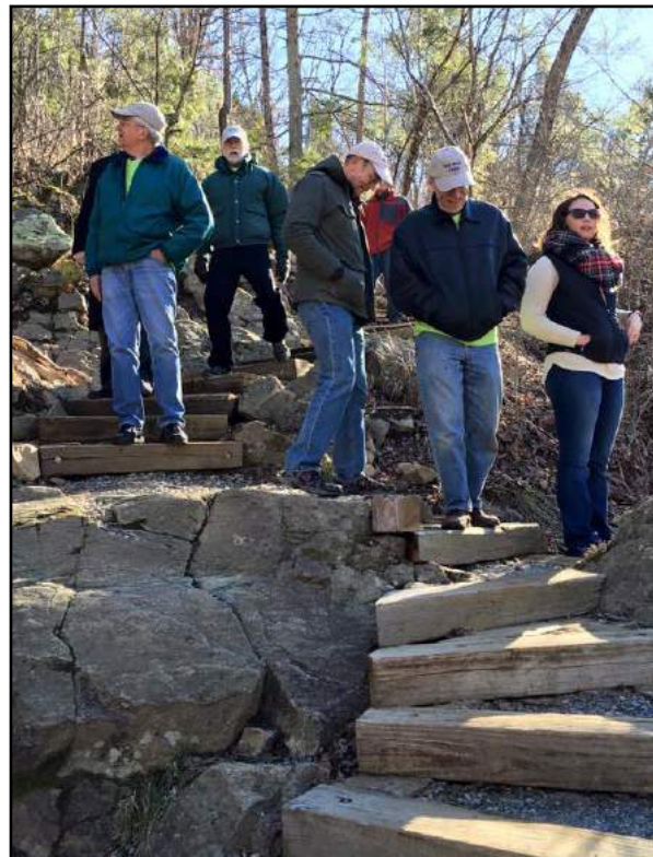
Volunteers built over 200 steps to provide access from the Blue Ridge Parkway to the Roanoke River.
